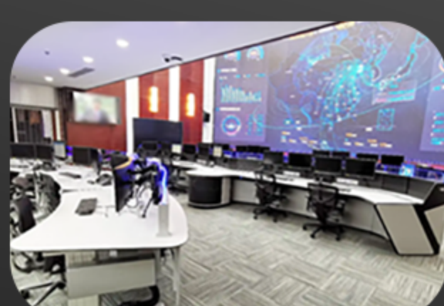
CONTROL AND COMMAND CENTER
